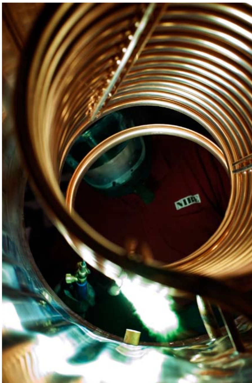
Copper is the commonest choice of non-corroding material on the Swedish and Dutch markets.
